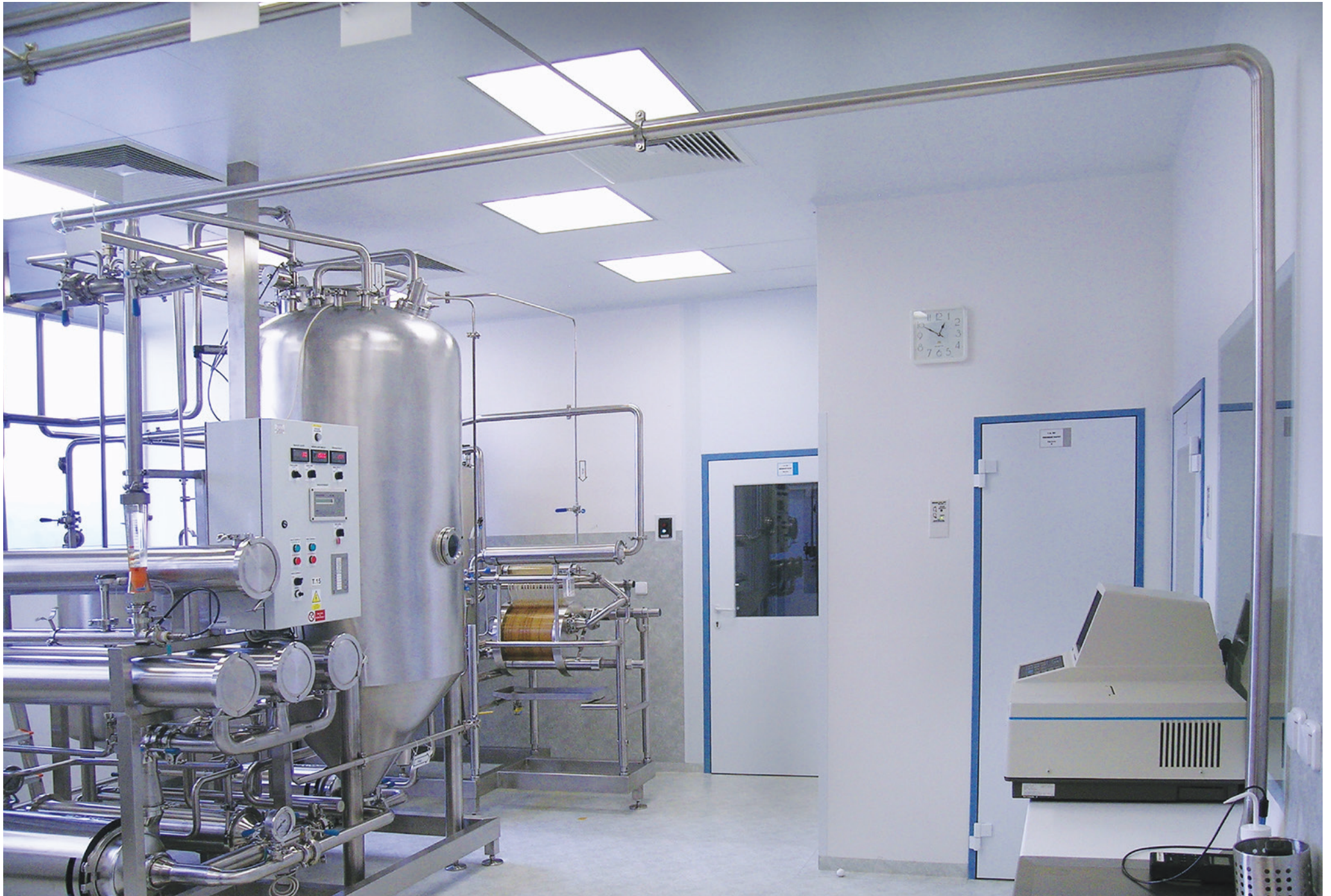
Completion of CONTIPRO a.s. Facilities – Stage II; Contipro a.s.; Ústí nad Orlicí, Czech Republic; 2006
