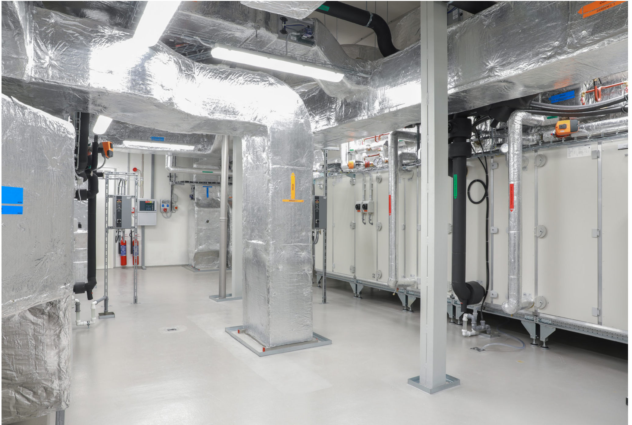
Construction Work and Extension of Building No. 3 for the Production of Hormonal Preparations; Bioveta, a.s.; Ivanovice na Hané, Czech Republic; 2020
