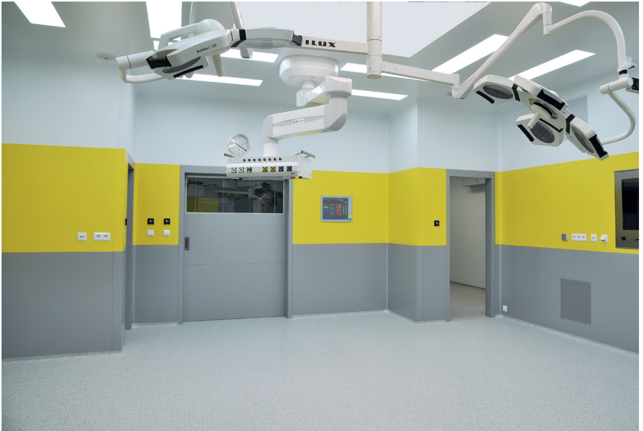
6 operating theatres and background | Hospital Uherské Hradiště | Czech Republic | 2014
