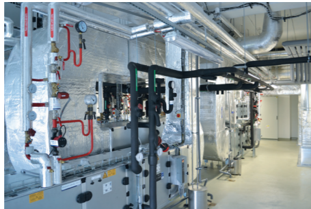
HVAC&R (heating, ventilation, air-conditioning and refrigeration) ⑤
